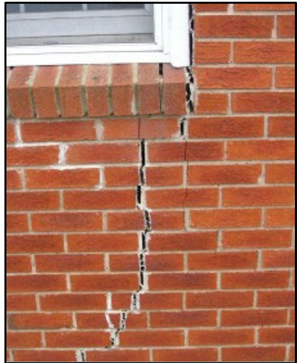
Figure 4.5. Cracked wall from a shifting foundation
