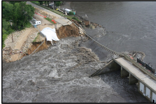
Figure 4.1. Dam Failure at Lake Delhi
